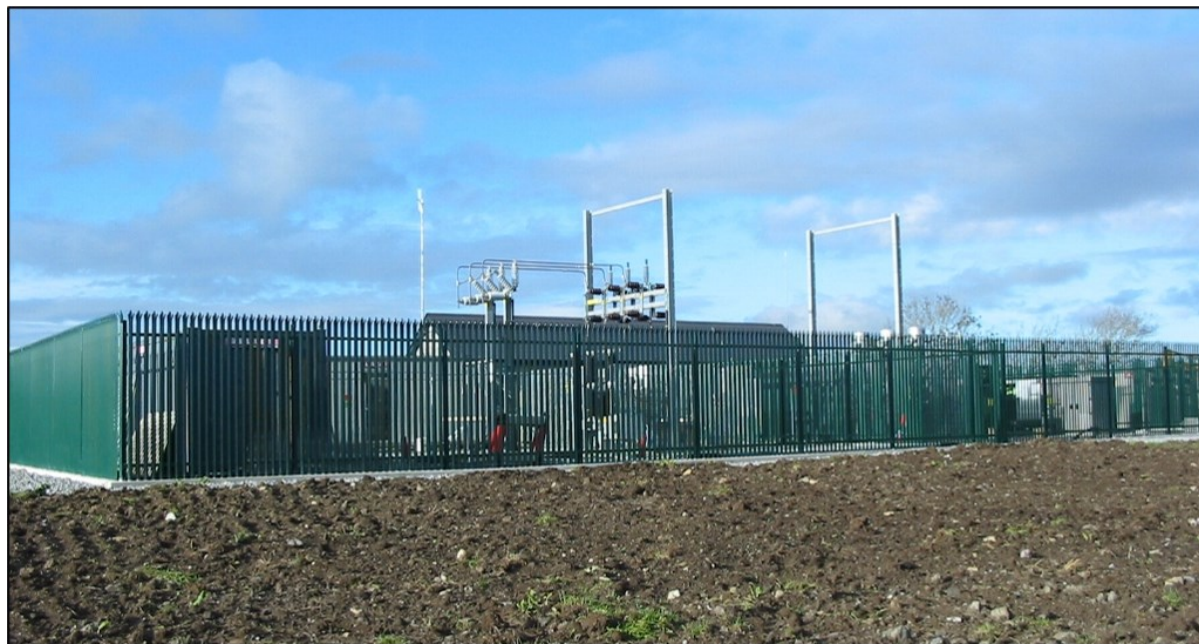
Figure 4-8: Example of Substation Compound
