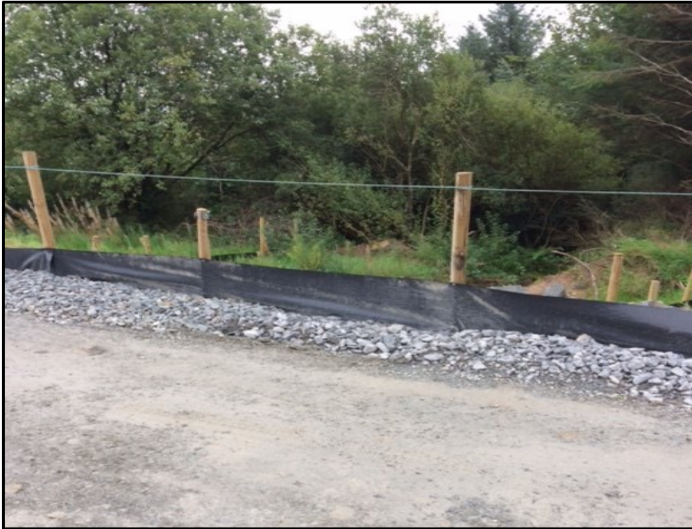
Figure 7: Dirty water containment at watercourse crossings
