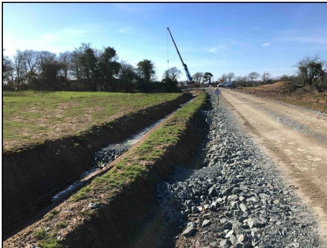
Figure 4: Separation of Clean and Dirty Water Drainage on A Wind Farm Site
