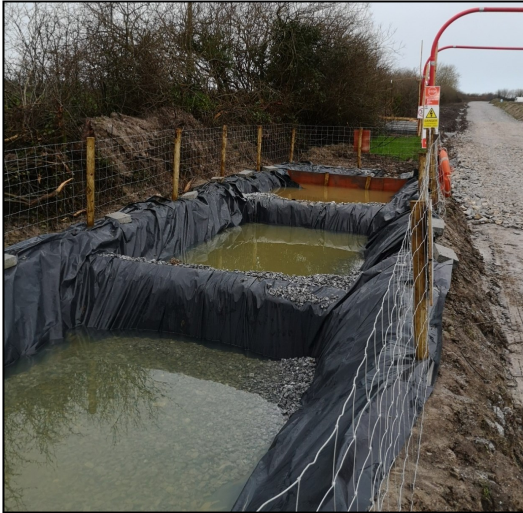
Figure 10: Multi-tiered settlement pond with stone filter
