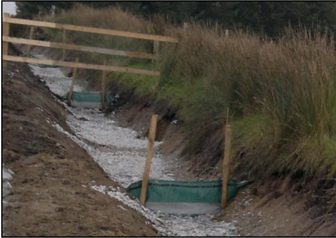
Figure 12: Example of a silt fence used in conjunction with check dams along trackside drainage channels
