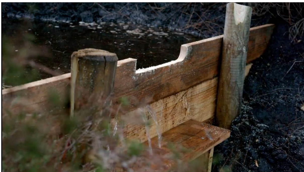
Plate 2: Wooden dam partially blocking drain.
