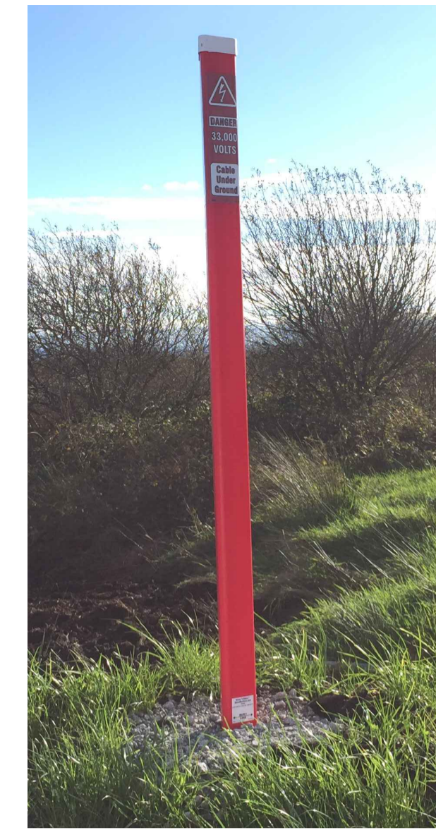
Cable Marker Post
