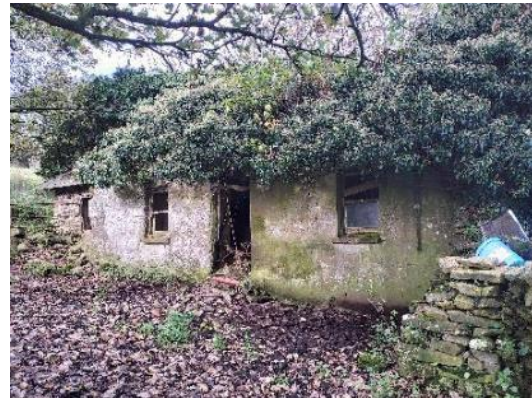
Plate 19: Derelict structure present east of proposed Turbine 7 displaying 'low' suitability for roosting bats
