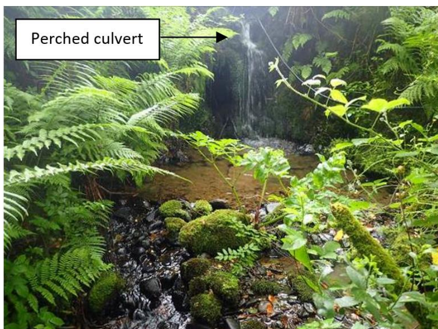
Plate 8. A perched culvert that likely limits the upstream passage of trout located at Site 2 on the 1 st Order Glennagross Stream, a tributary of the Crompaun Stream.
